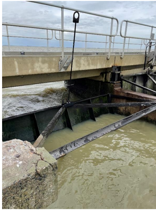
Radial gate at Ewe Island barrage (K. Williamson, DEW)
