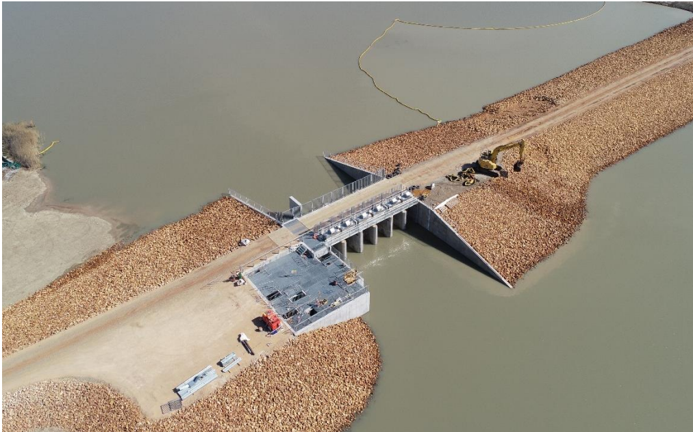
Figure 1: Newly constructed environmental regulator on the Pike Floodplain (Source: Dan Haines, SA Water)
